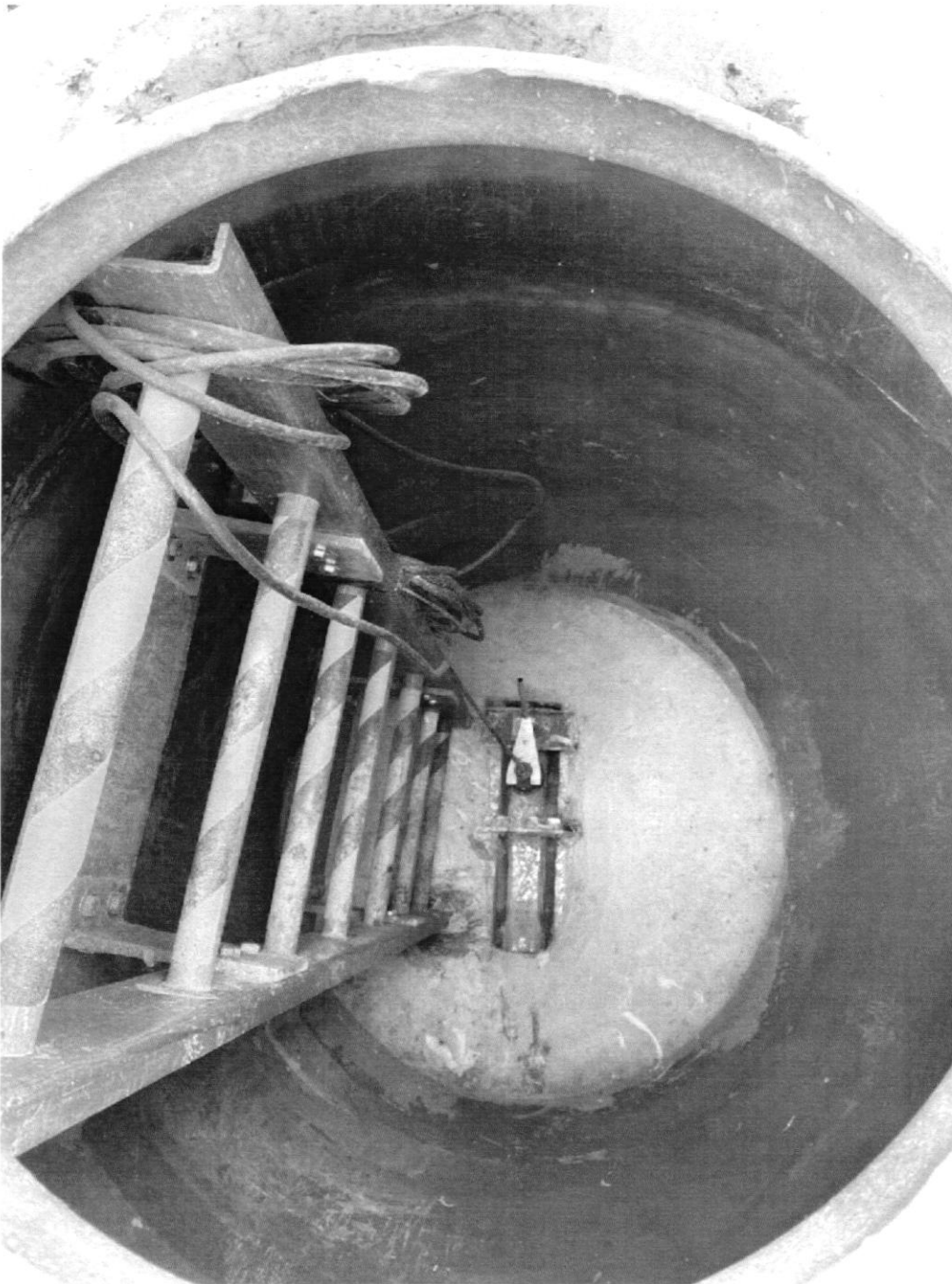
Swan Manor's vault shows no signs of overflow, and approximately 10 gpm (1 inch) flowing through the flume.
